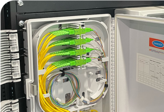
Excellent cable management utilising the double sided cassette ensure network maintenance, adds, moves and changes are simple to perform
